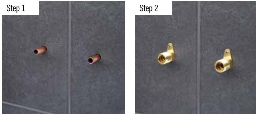
Step 1 Finish the wall leaving the pipe stubs protruding at least 50mm.
